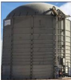
Figure 15. Picture of typical gas bladder
