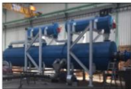
Figure 12. Photo of typical low temperature pyrolysis unit.
