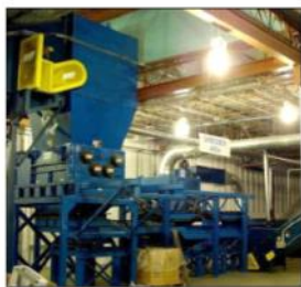
Figure 7. Photo of a typical Moisture/Discharge system.
