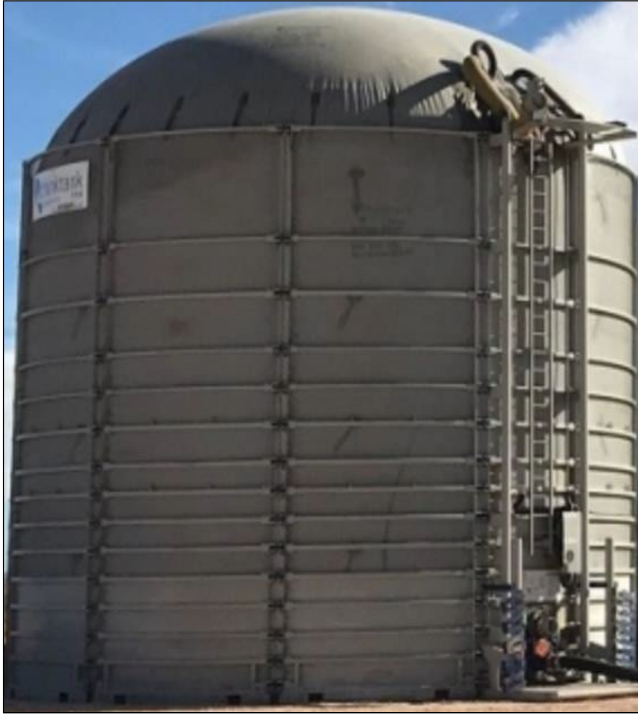
Figure 14. Picture of typical gas bladder
